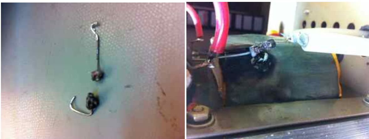
Failed resistor and transformer damage
