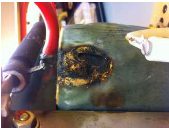
Transformer case charring
